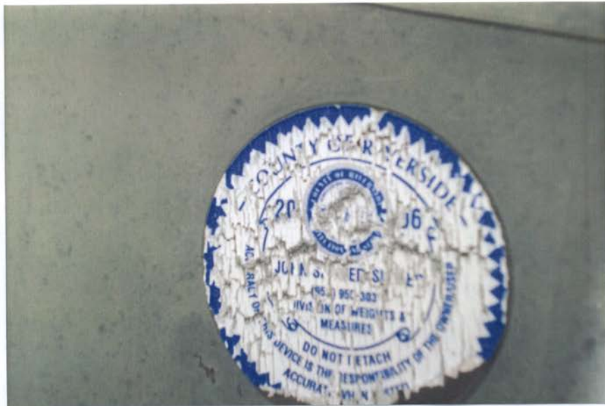
BLYTHE AIRPORT – 2006 WEIGHT AND MEASURES CERTIFICATE SEAL ON AVIATION GAS FUEL PUMP ATTACHMENT "B"
