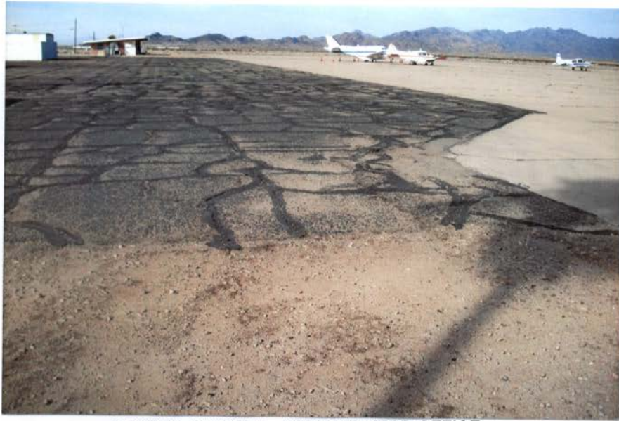
BLYTHE AIRPORT – ASPHALT NEAR OFFICE ATTACHMENT "A"
